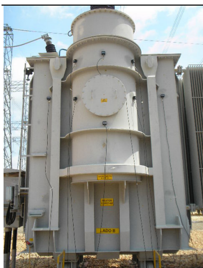
Figura 7 – Reator monofásico 500 kV / 50 MVA
